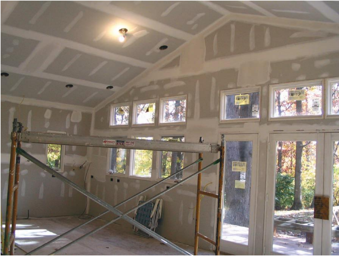
FIGURE 14.24 Gypsum board has been screwed to the wood framing in this new kitchen addition and finished out with taped joints. After some surface sanding, it is ready for paint.
