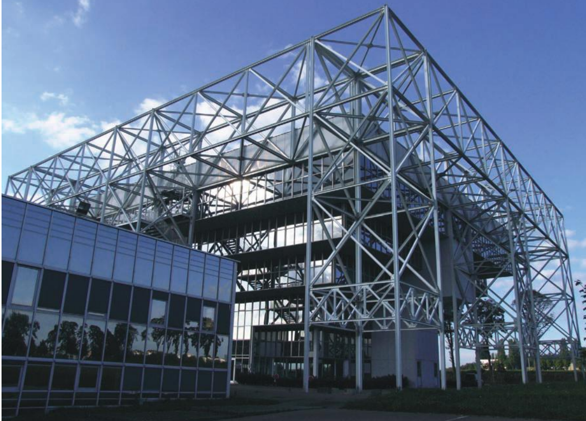
FIGURE 14.8 Space frames, such as this one in France, can span large areas with a minimum of supporting columns. Courtesy of Jacques Mossot ( www.structurae.de )
